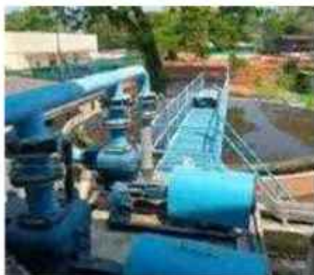
500 KLD STP at Kozhikode medical College
