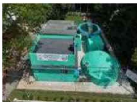
360 KLD STP at General Hospital, Thrissur
