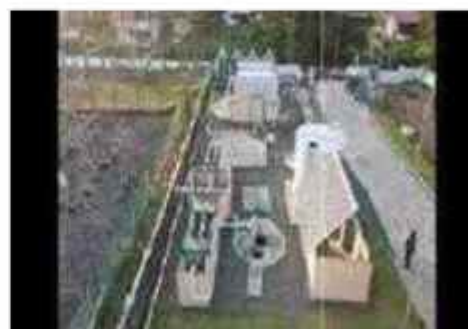
1 MLD CSTP at Pedanappalam, Kannur
